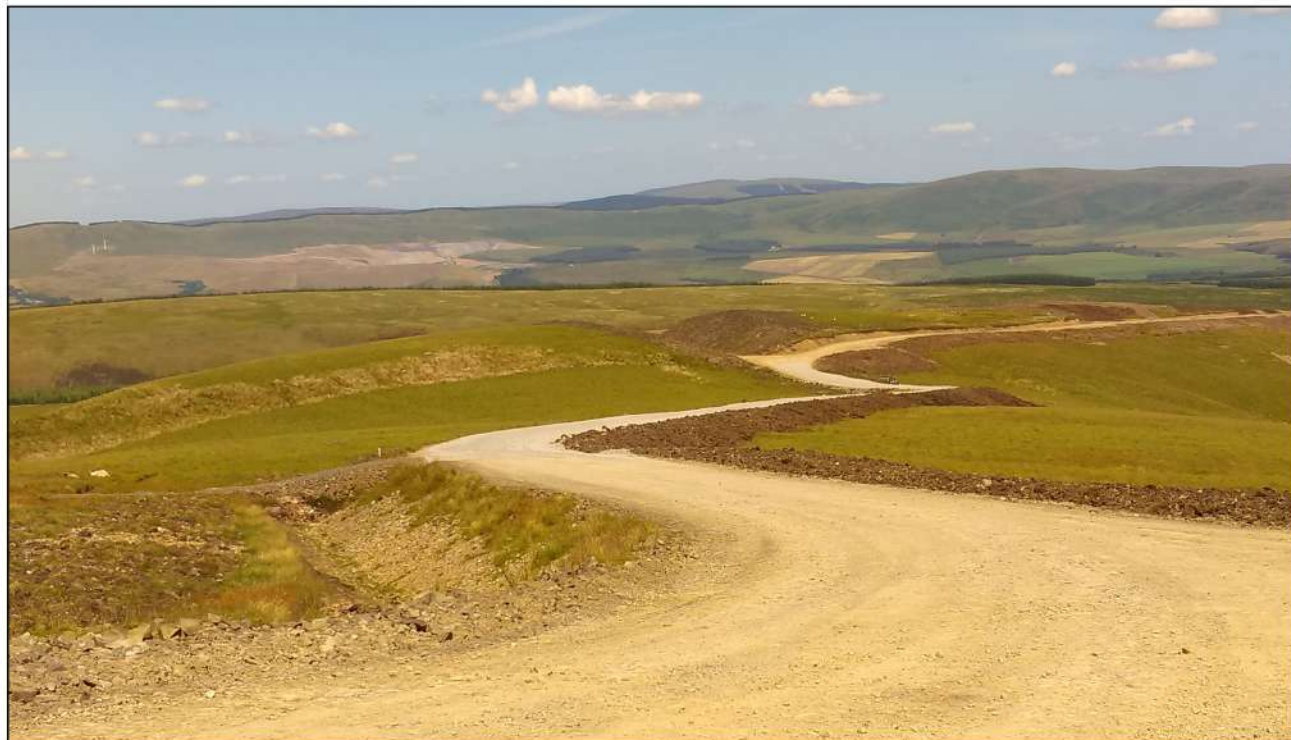
AI Plate 2.4c - Completed floating access track at Sanquhar Community Wind Farm.
