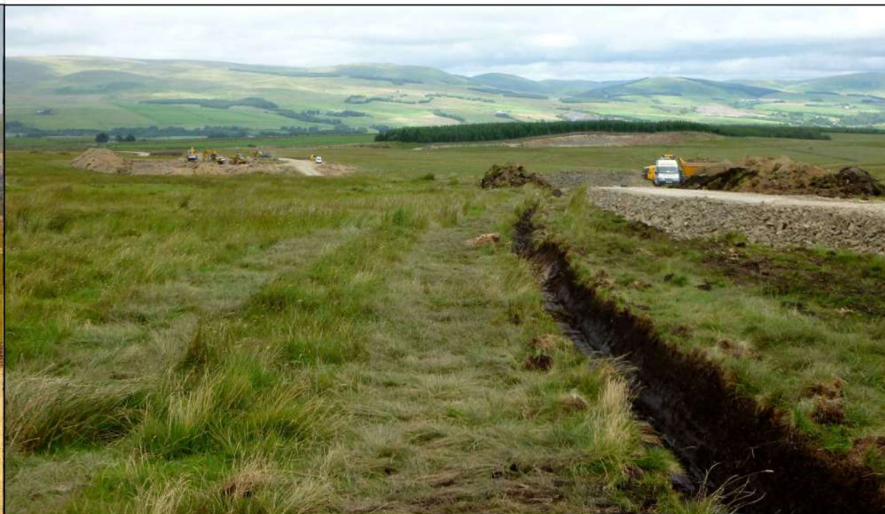
AI Plate 2.5 - Drainage Ditch Adjacent to access track at Sanquhar Community Wind Farm.
