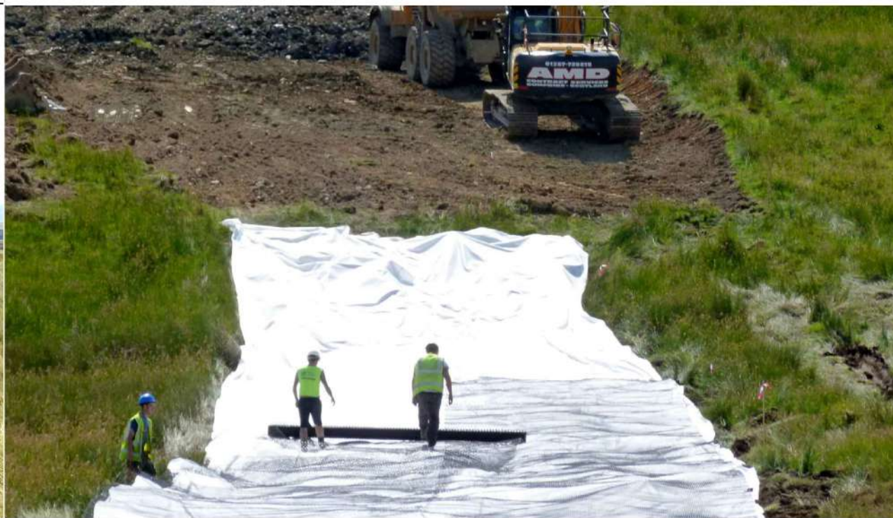
AI Plate 2.4b - Floating track into cut track transition at Sanquhar Community Wind Farm.
