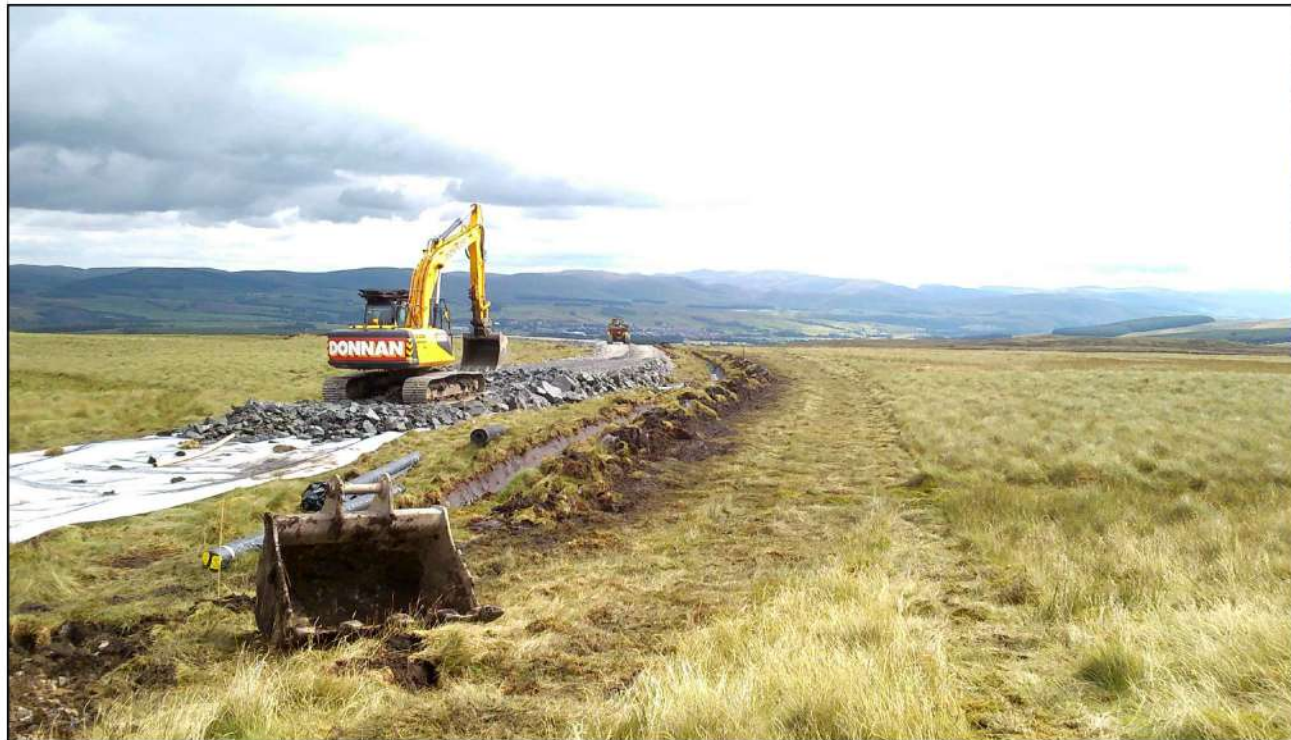
AI Plate 2.4a - The construction of a floating road at Sanquhar Community Wind Farm.
