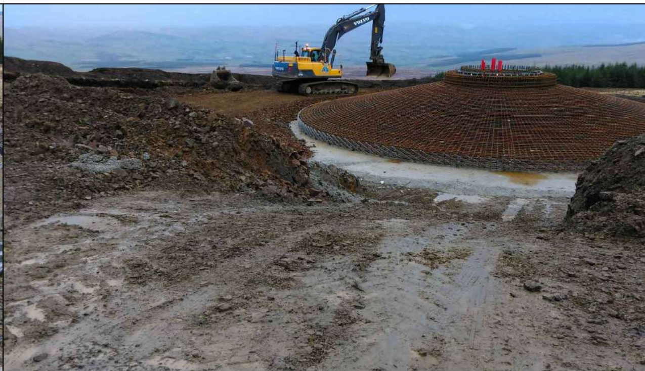
Plate 2.2b - Steel reinforcement which forms the turbine foundation at Sanquhar Community Wind Farm
