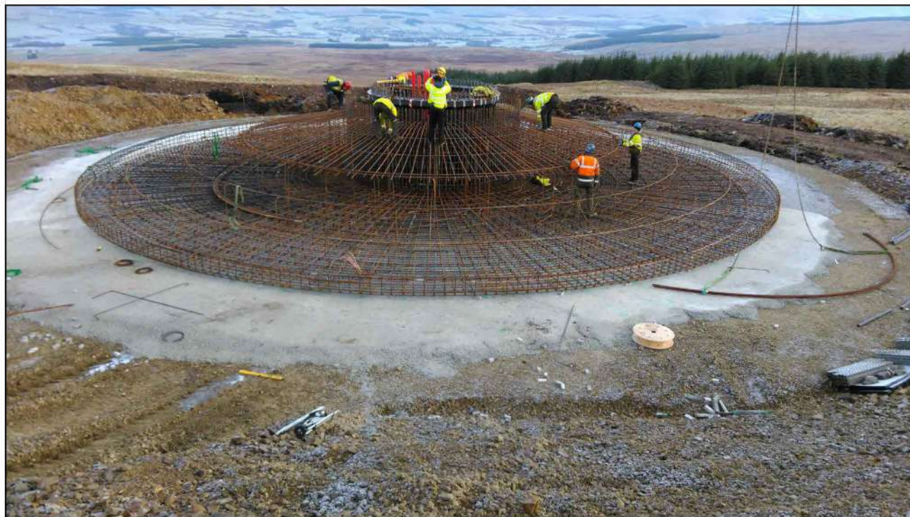
Plate 2.2a - Steel reinforcement which forms the turbine foundation at Sanquhar Community Wind Farm
