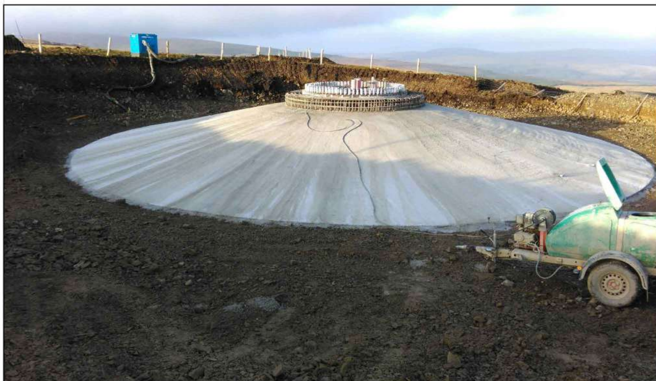
Plate 2.3a - Concrete finishing to a turbine foundation before backfilling at Sanquhar Community Wind Farm
