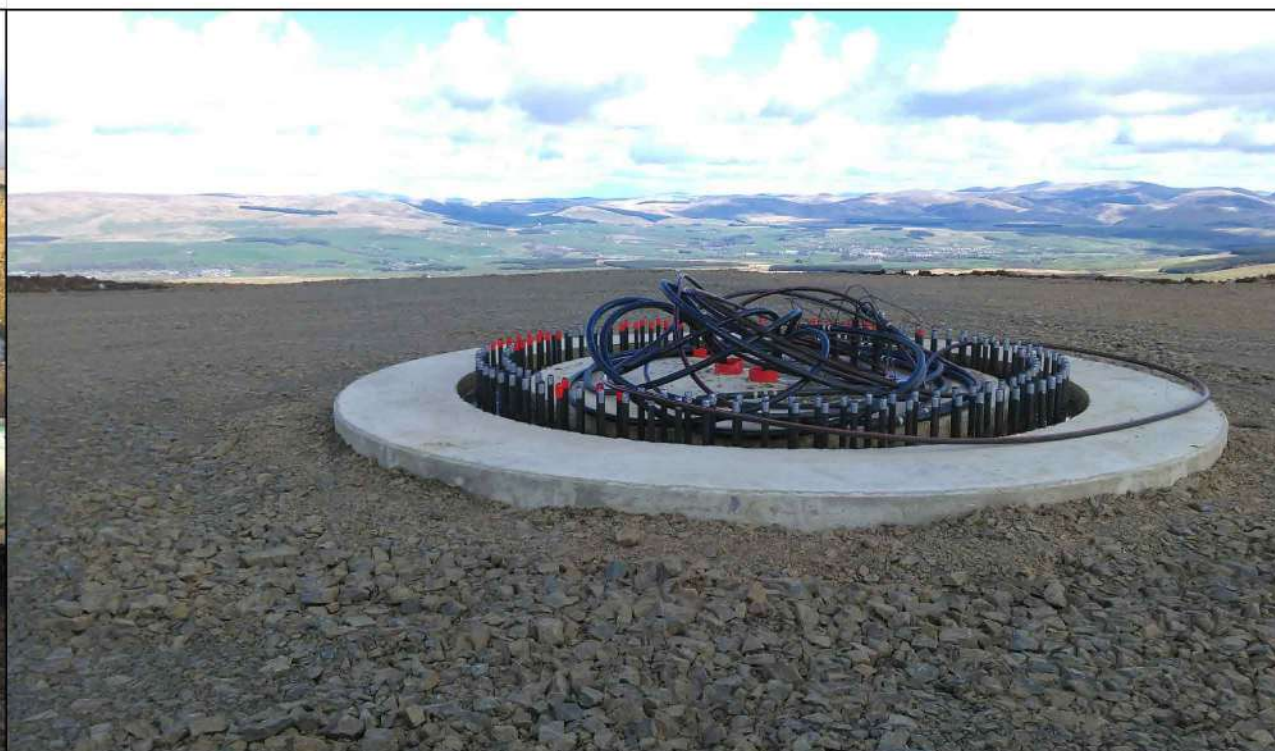
Plate 2.3b - Concrete finishing to a turbine foundation after backfilling at Sanquhar Community Wind Farm
